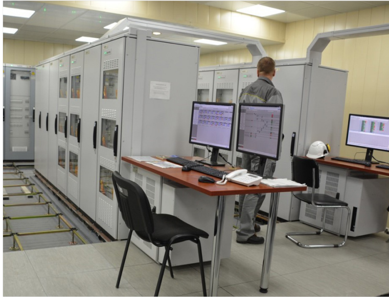
Digital Safety Systems Require Fewer Equipment Racks, Reducing the Total Data Center Footprint
